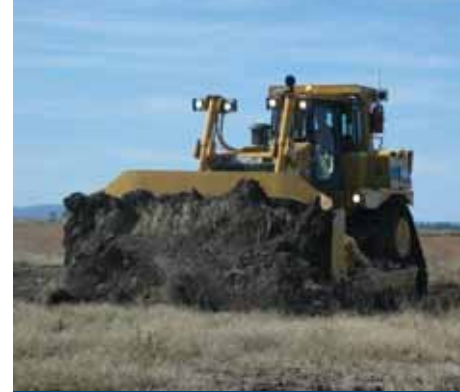
Above: A dozer creating a safety bund around the new Dawson pit.
