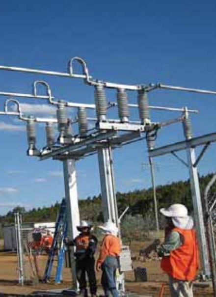
Above: Construction of the coal bed methane driven power station at Capcoal.
